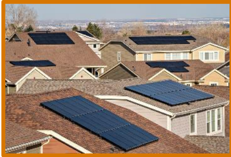
Rooftop Solar Panels
